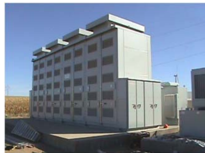
Xcel Wind-to-Battery Project Luverne, MN 2008 1,000 kW Sodium Sulfur Duration: 7 hour at 1MW
